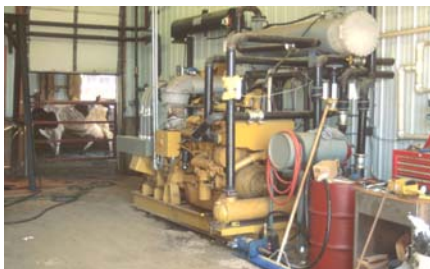
A generator on a diesel motor converted to run on methane from the digester provides electricity for the Haubenschild farm operations, Princeton, MN.
