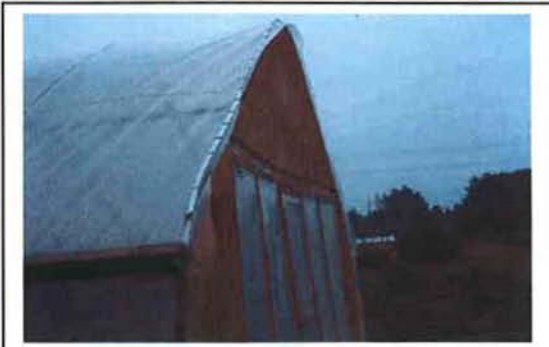
Figure 5. End wall before reinforcement.
